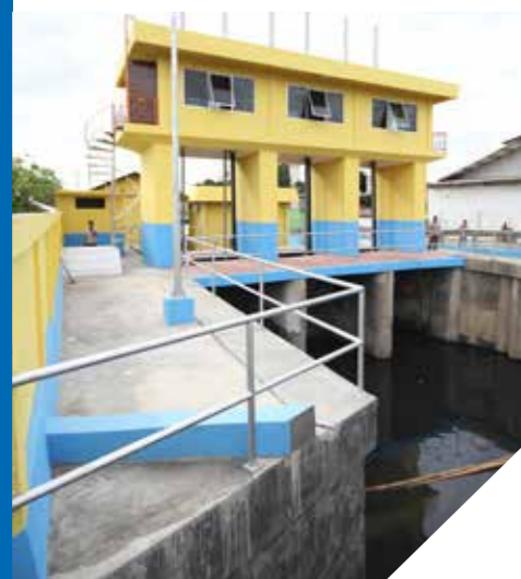
The Grundfos Pump Gate solution was the most suitable for Poglar, considering the limited land area required and the flow conditions from the Angke River.
